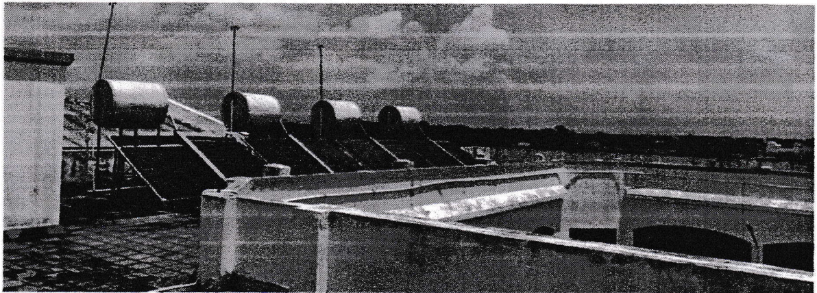
Solar Water is Installed in College Staff Quarters & Hostel
