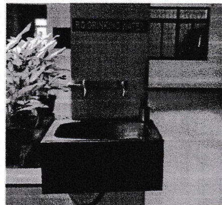
Purified Water Unit Installed In all Blocks
